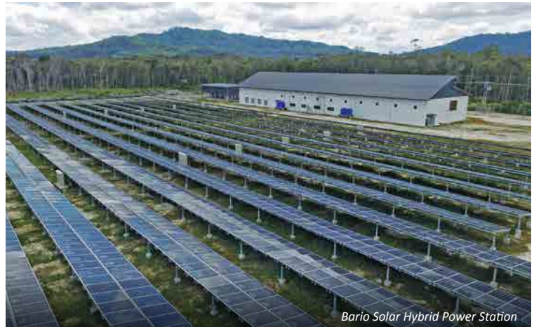
Bario Solar Hybrid Power Station
