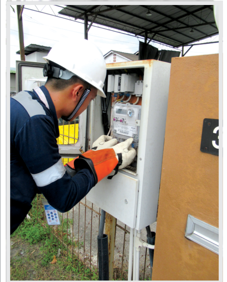
Smart meter installation
