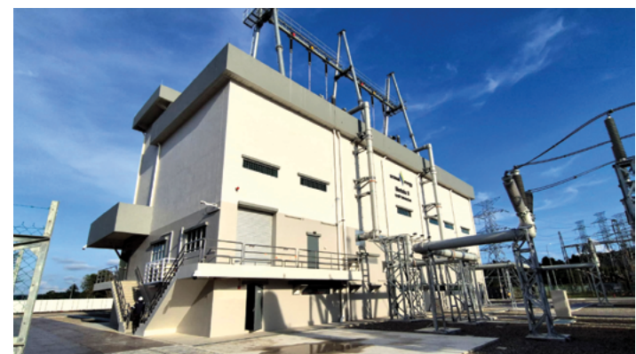
Bintulu B 132kV Substation
