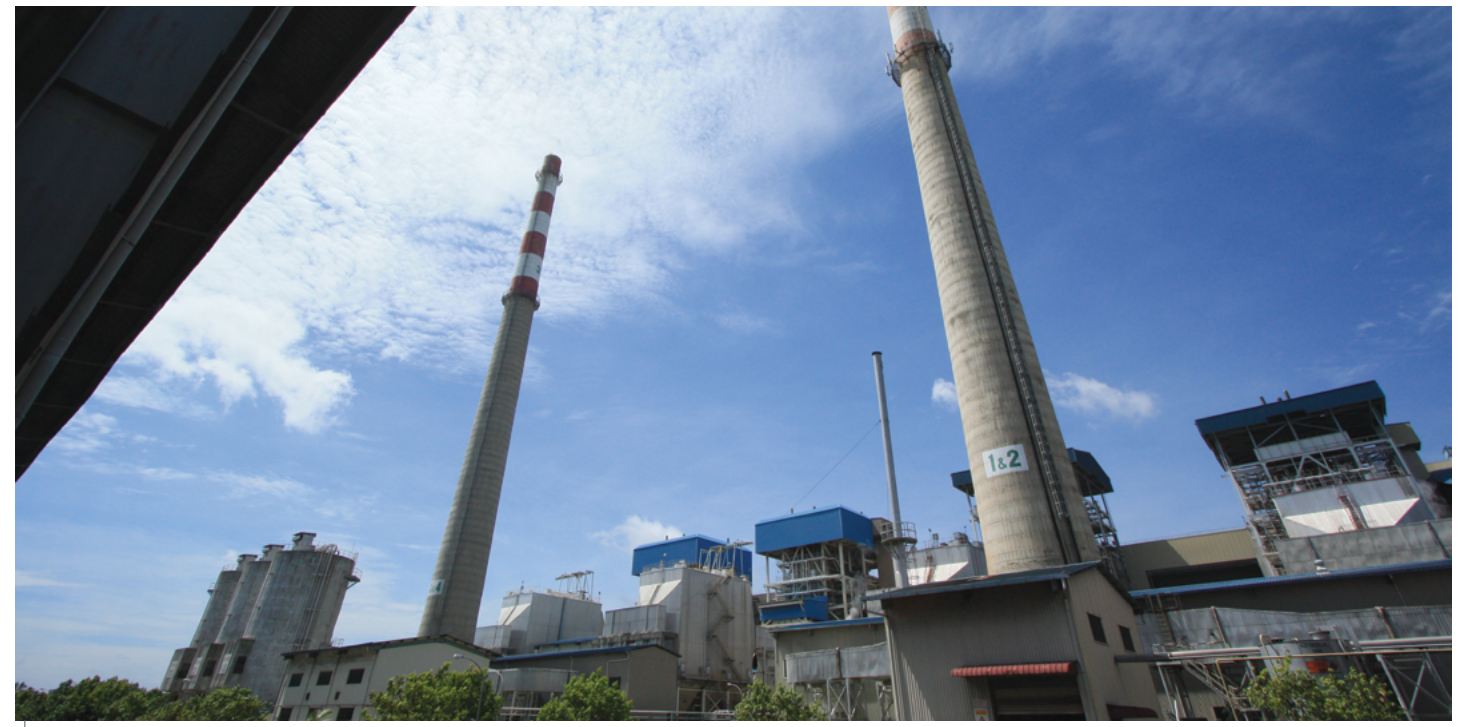
Sejangkat Power Corporation Coal-Fired Power Plant
