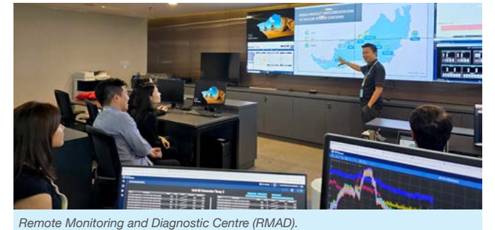
Remote Monitoring and Diagnostic Centre (RMAD).
